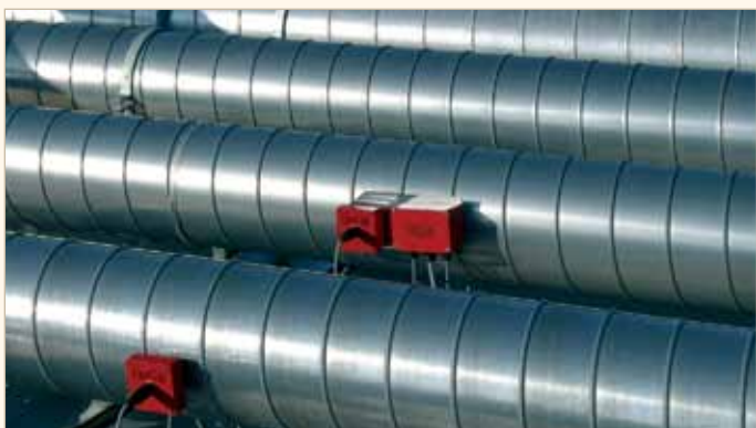
Extraction system with spark detectors
